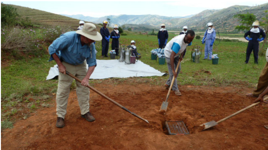
PMI AIRS project staff set up a mobile soak pit in Madagascar.
